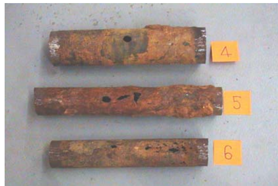
Figure 6 Failed steel pipe sections
