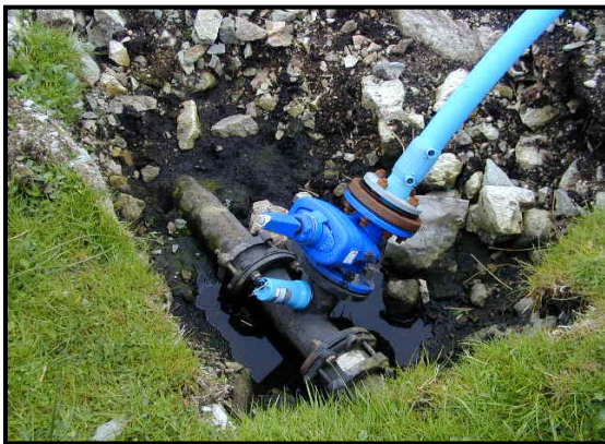
Figure 6 Leak Noise Correlation Pods
