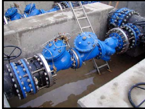
Figure 17 two units of two-step pressure control system (PCVs)
